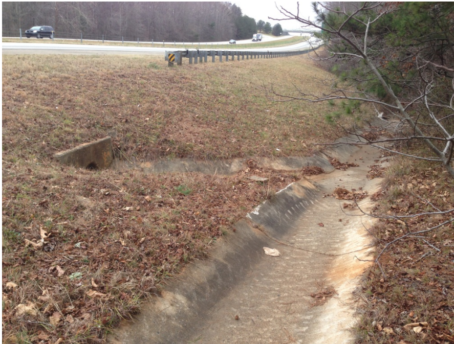
Photograph 3.4.4. Rural interstate example of surface runoff collected by paved ditch and connecting piping from median drainage.
