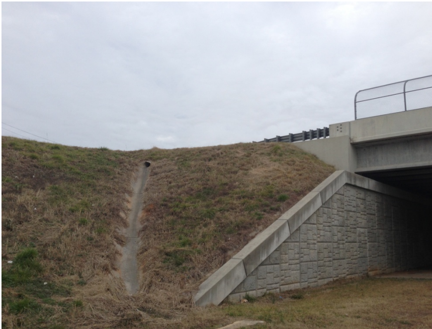
Photograph 3.4.6. Example of rural interstate overpass bridge deck drainage to abutment for collection and piped discharge to paved ditch and subsequent runoff.
