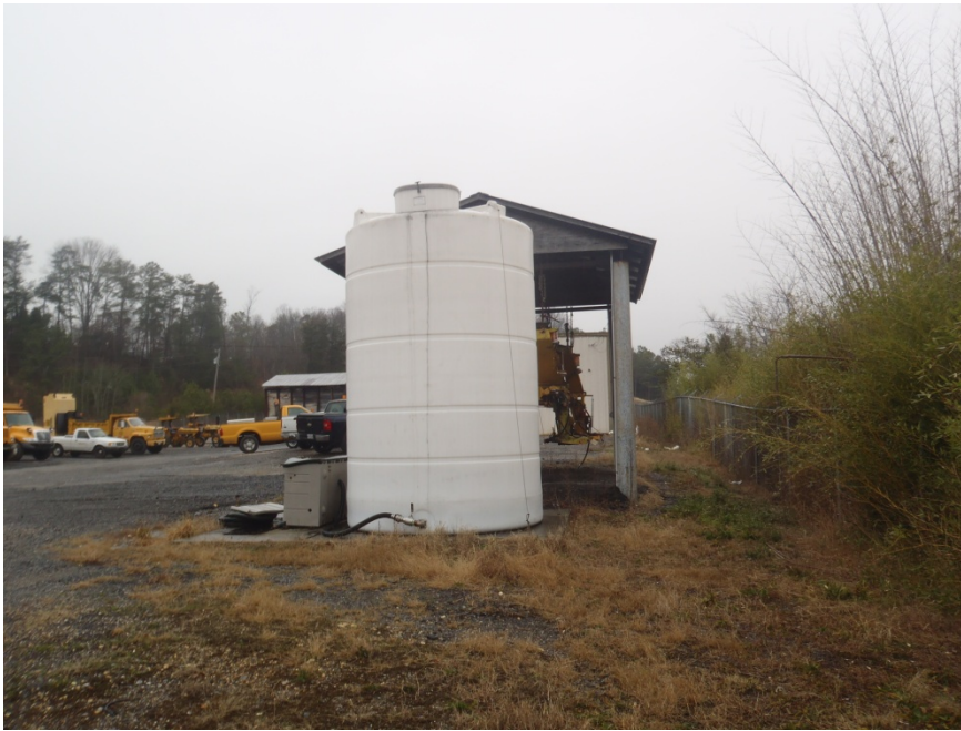
Photograph 3.2.15. A typical brine solution preparation and storage tank.
