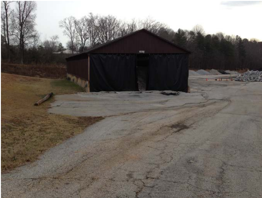
Photograph 3.2.13. A typical older wood timber Salt Barn with end curtains at a Maintenance and Storage complex.
